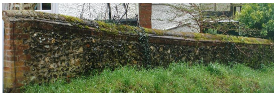
Picture 23. Wall of brick and flint construction to front of Clare Cottage Snow End House .
