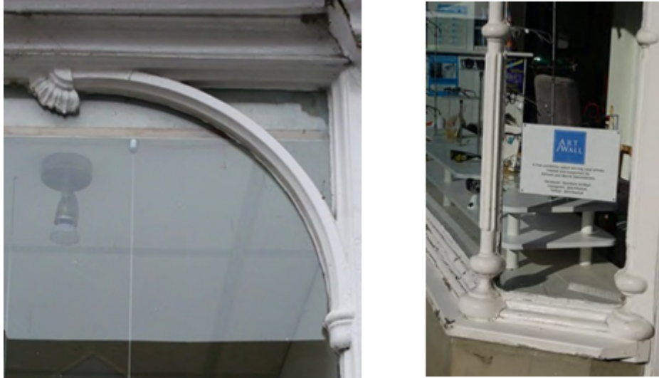
Figure 34 - An interesting Edwardian decorative glazing bar and a moulded mullion from the late-19th century.
